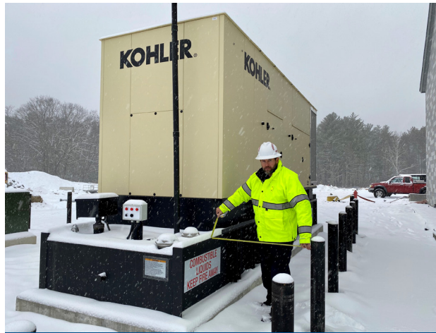
State Building Inspector, Ryan Brautovich, with the Fire Marshal's Office – Bureau of Building Safety and Construction (BSC), performs a final inspection on a commercial generator to ensure proper code compliance.
